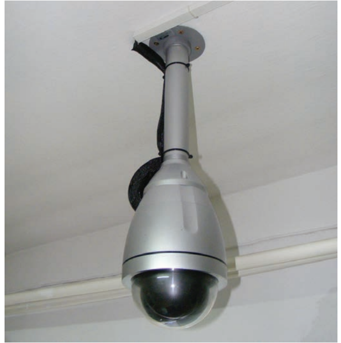
Fig. 2. Ceiling mounted camera in outlying hospital's resuscitation room operated from the command control room
